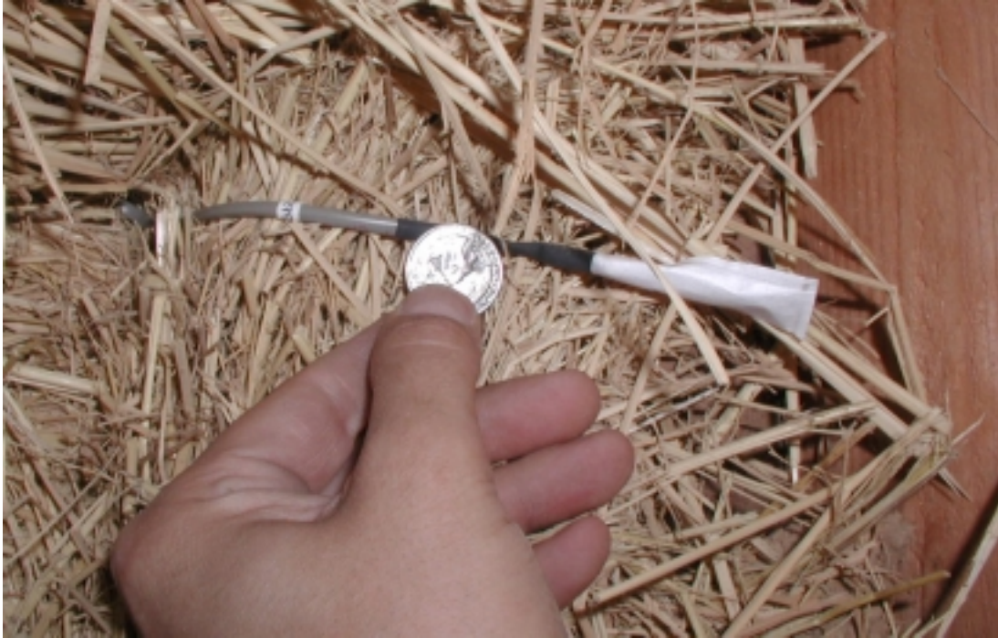
Figure 2.4: Relative humidity and temperature sensor installed in SB
