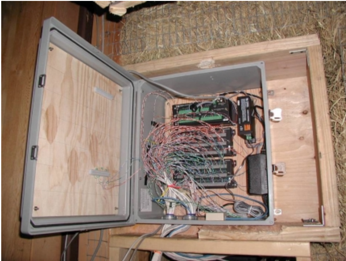
Figure 2.6: Barrel Room Data Acquisition System
