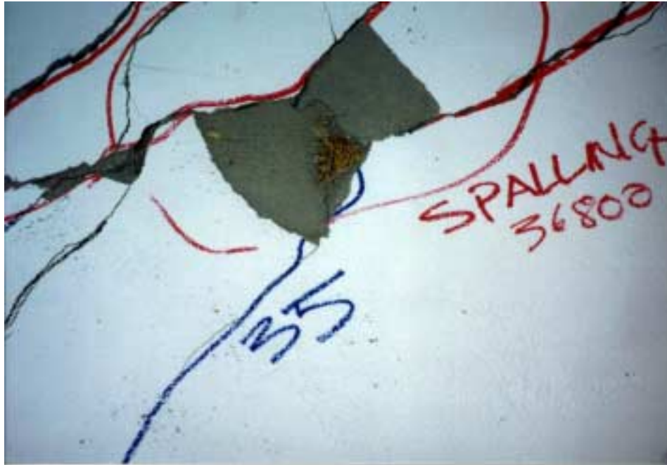
Figure 14 – Spalling on left face
